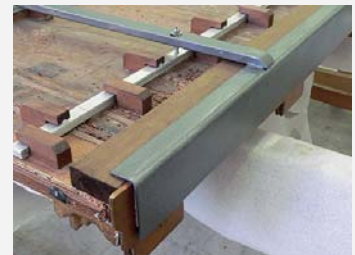
Detail of the wooden framework and of the support base after the restoration.
