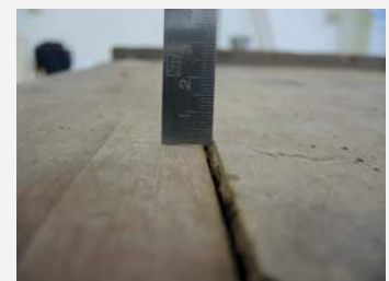
Detail of unevenness along a crack.
